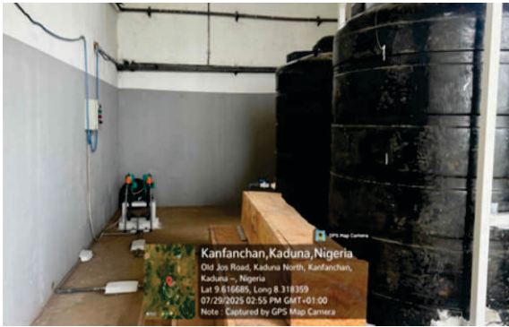
The automated chemical dosing machines
