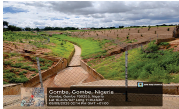
Gully head after the intervention.
