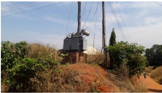
Transformer behind AA Suite Health Care
