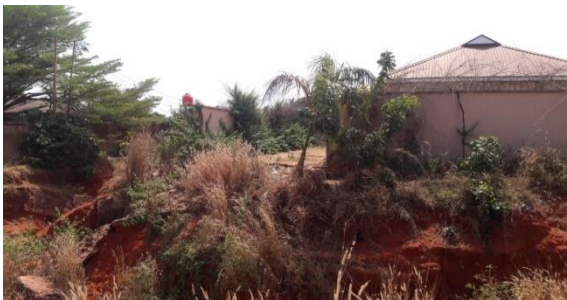
Dilapidated AA suite Fence
