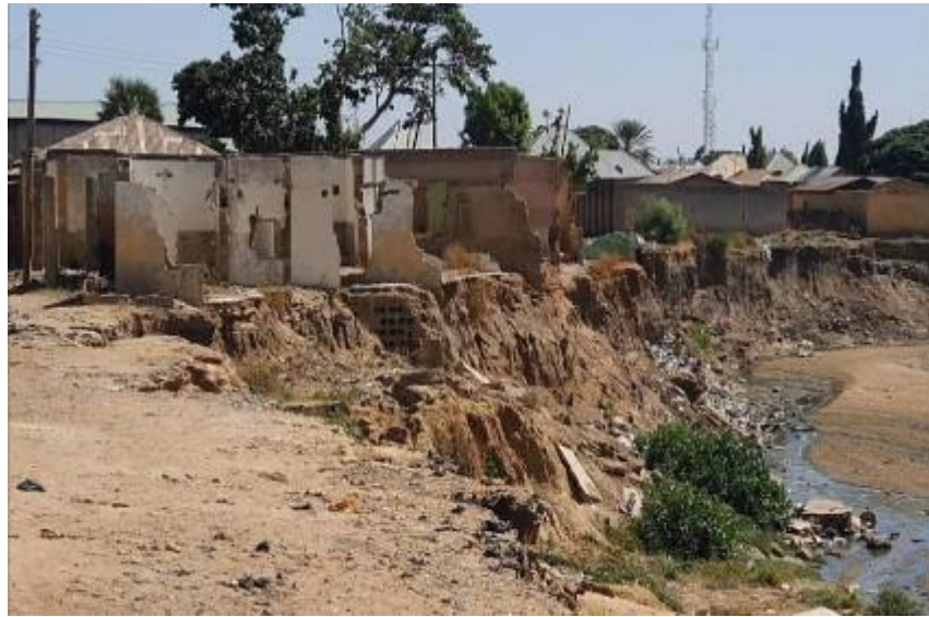
Plate 2. 1: Midstream with serious erosion devastation impact , Source: RAP Survey 2024
