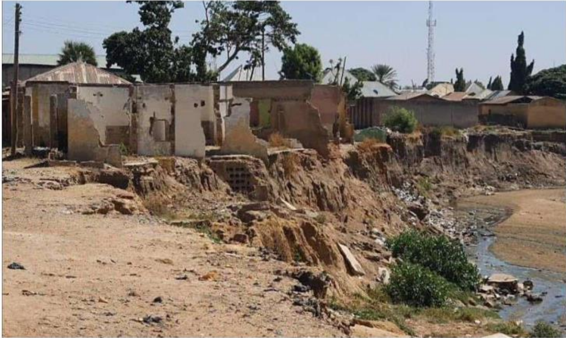
Plate 1: 1: Channel bank erosion showing properties (houses) at risk.
