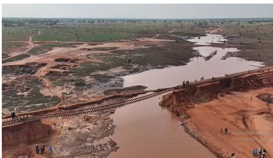
Figure 1.3: Damage to Rail-Line Embarkment in Mokwa Due to Flash Flood
