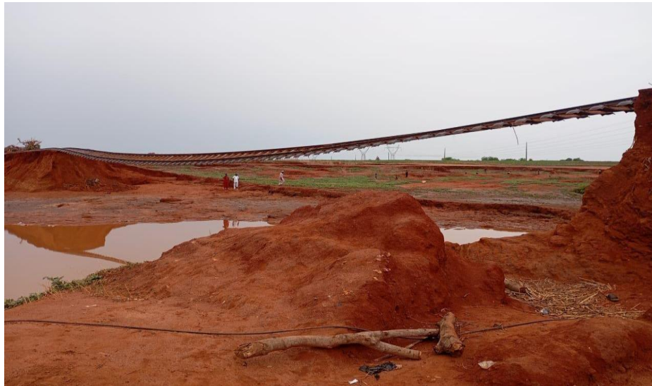
Figure 1.4: Destruction of Rail-Line Embankment by the Flash Flood
